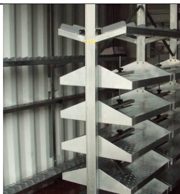
Detail of racks
