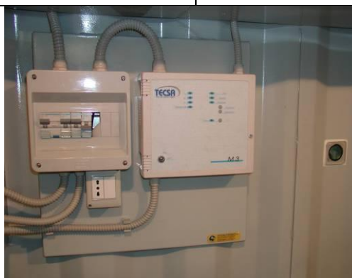
Detail of electrical panel (interior) and alarm box
