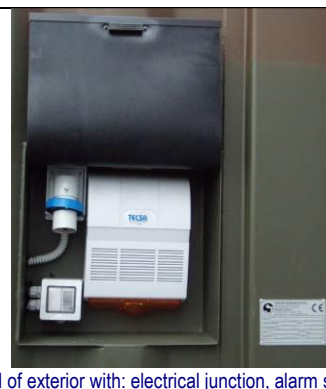
Detail of exterior with: electrical junction, alarm switch – internal light switch and siren with flashing light
